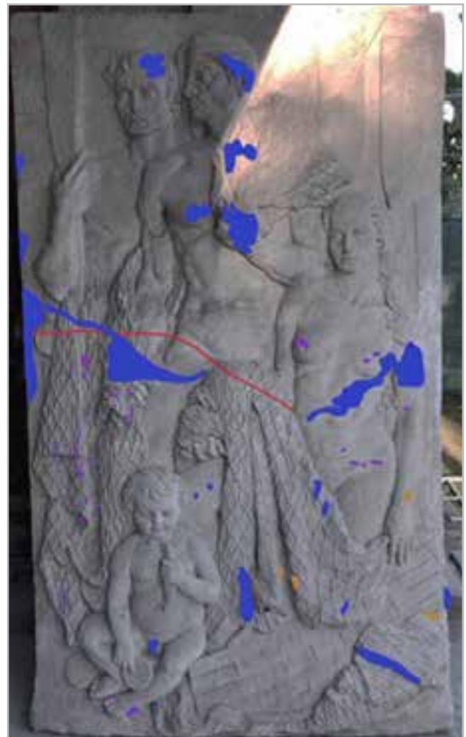
Figure 2.- Pathology Mapping (Blue: subsequent interventions; Purple: paint droplets; Orange: oxidation stains; Red: Cracks).
