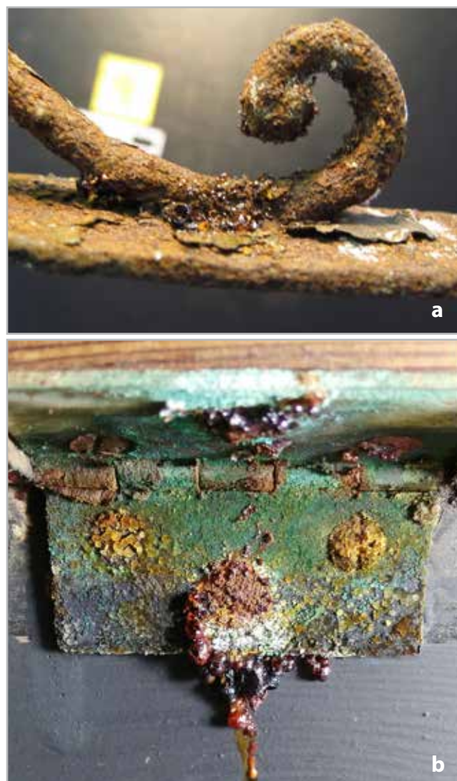
Figure 4.- a: condition of one of the iron brackets that supported the glass shelves. b: one of the most corroded copper hinges (M. Pèrez and A. Casalod).
