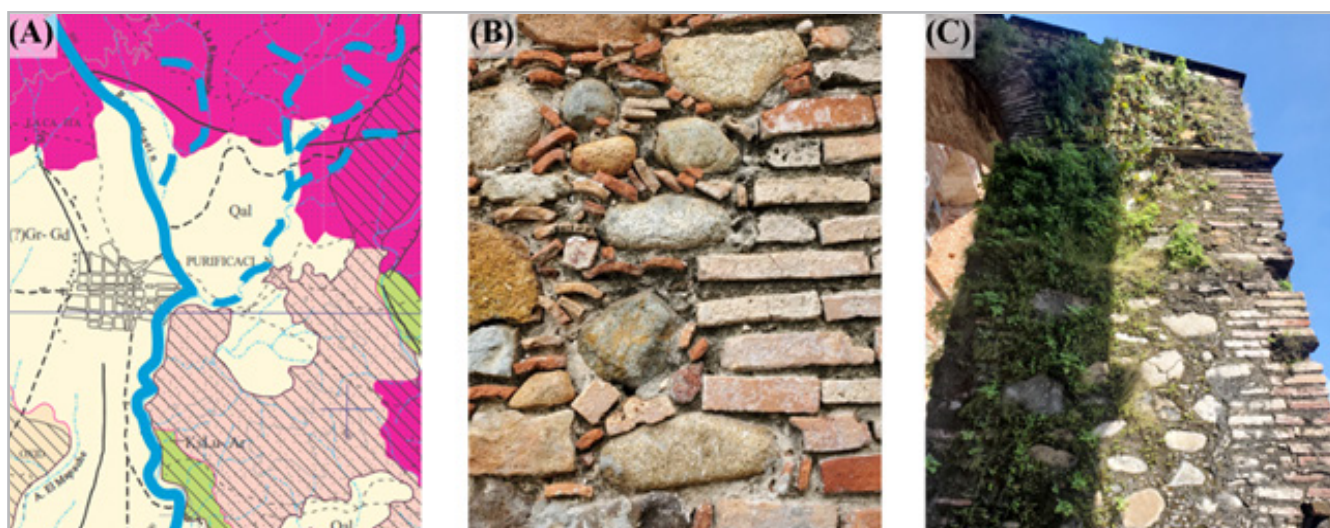
Figure 7.- (A) Pluvial causes. (B) Rounded-edged stones on the second buttress in front of the gate. (C) First buttress behind the tower, damage mainly to bricks and mortar.
