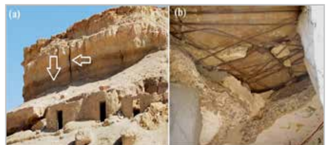
Figure 4.- (a) geotechnical defects in the rock structure of the areas, (b) failure of the ceiling of the tombs and the iron bars used in old restorations of the tombs.
