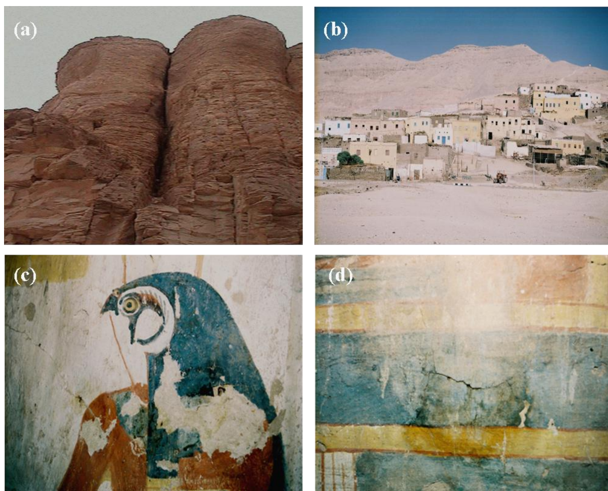
Figure 1. (a) View of the Theban Mountain, El-Qurna necropolis. (b) View of Qurnet Marai necropolis. (c) Loss of the paints and painted flakes express the state of conservation of the wall paintings at Tomb of Ameneminet , No. TT277. (d) Different cracks spread over the painted surfaces.
